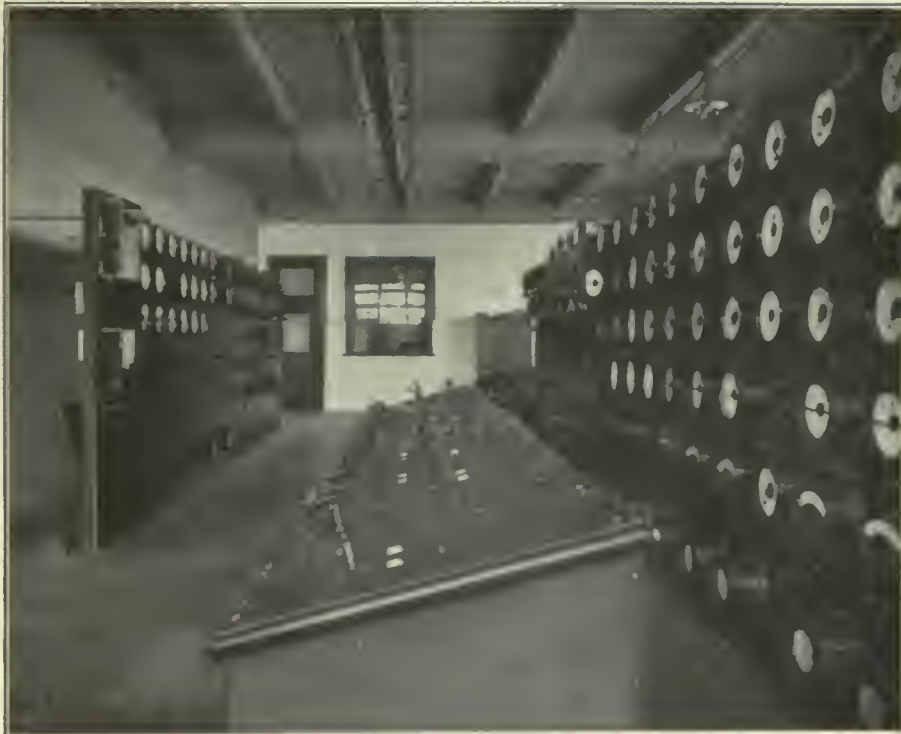
FIG. 490. POWER STATIONS. Bench Board in Switching Gallery, Power Station of the Pennsylvania Railroad at New York City.
